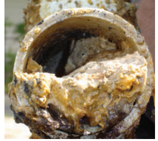
Grease clog inside a pipe.
